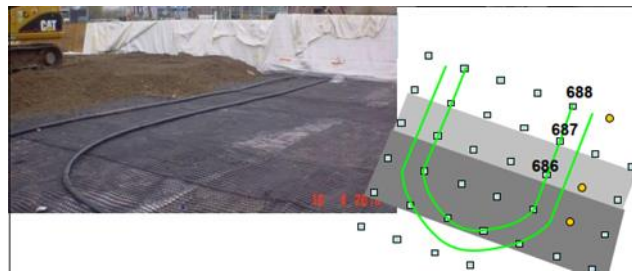
Figure 13. Example of monitoring arrangement
